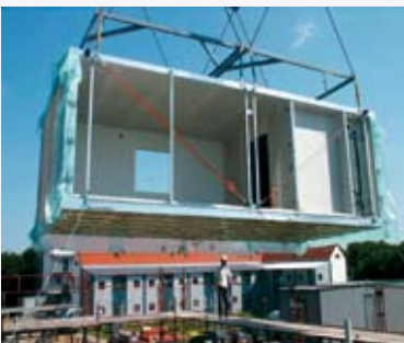
OpenHouse module during installation showing use of open sided modules with additional temporary posts
