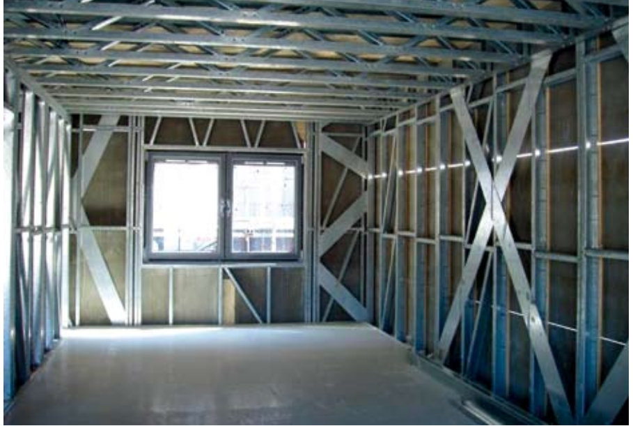
Figure 3.3 Lattice joists supporting gypsum screed used in long span floors Metek Building Systems
