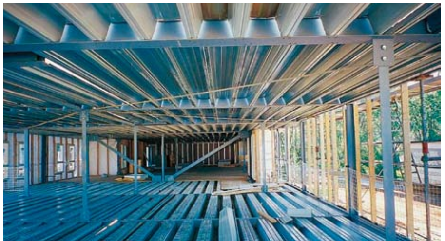
(Right) Intermediate floor showing wide open space for flexible arrangement of partitions and intensive use of steel elements
