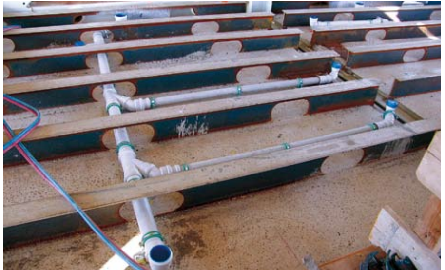
Figure 5.5 Inverted steel beams ( Slimline )
