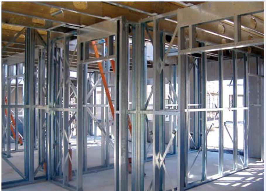
Figure 3.1 Floor systems using light steel joists supported on light steel walls Fusion Building Systems
