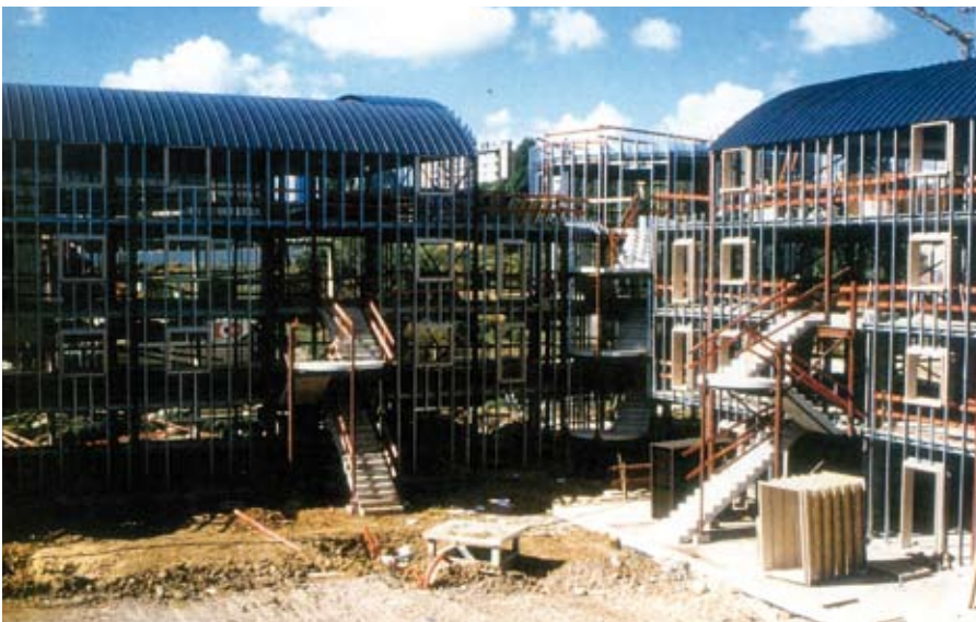
Figure 8.10 The PRISM system during construction: Steel frame, roof and external light steel walls ready to receive external skin
