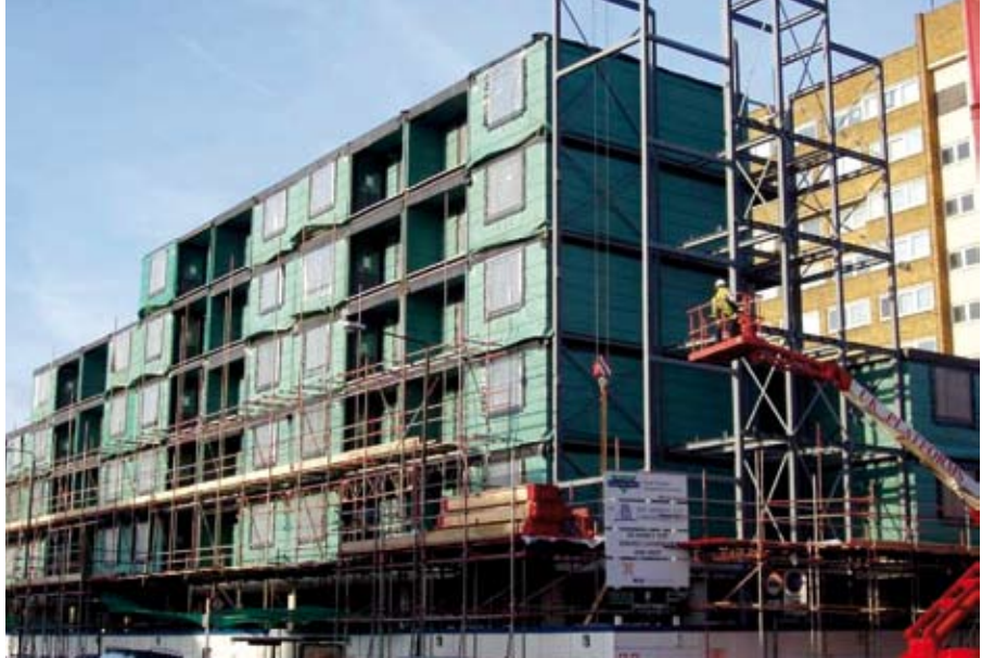
Figure 6.6 Modular building supported on a podium level and stabilised by a braced steel structure around the stairs
