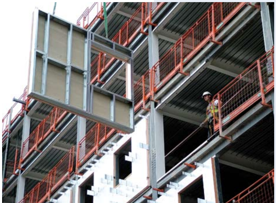
Figure 4.1 Installation of light steel infill wall in a steel frame Kingspan Architectural
